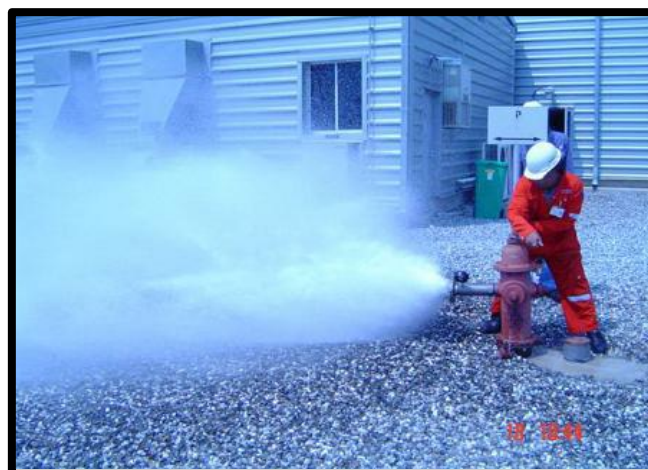
Hydrant Flow Rate Testing
